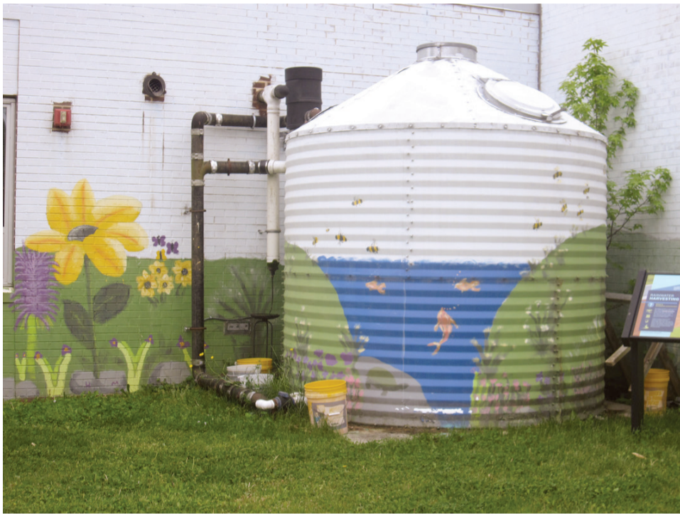
The school collects rainwater in two cisterns for reuse in their gardens.
